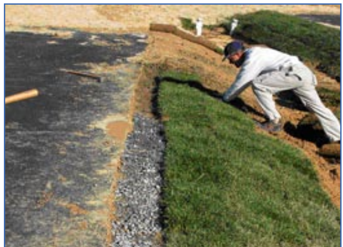
FIGURE 6. Installing a gravel verge and sod stabilizes the perimeter of bioretention cells and is highly recommended. The resulting filter strip shown here is 5 feet wide.
