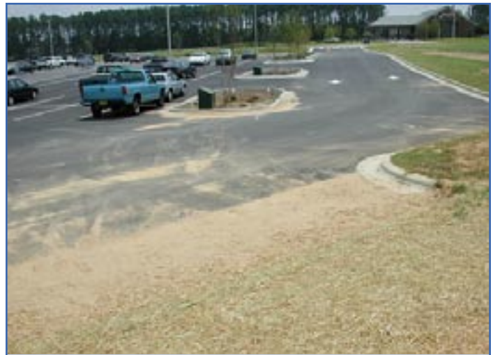
FIGURE 4. An out-parcel was not stabilized (foreground), leading to the clogging of the bioretention cell pictured next to the pickup truck. The trail of sediment from the out-parcel to the bioretention cell is clearly visible, as is the sediment eyebrow around the bioretention cell.
