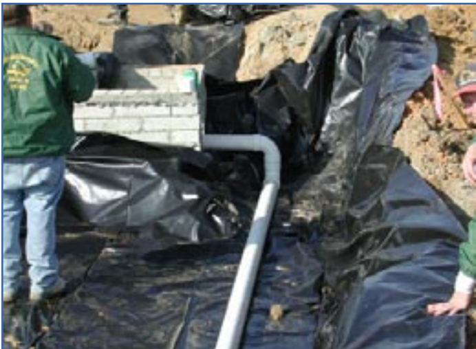
FIGURE 1. An Internal Water Storage Zone (IWS) is incorporated into a bioretention cell by forcing water to move “uphill” through the underdrain system.
