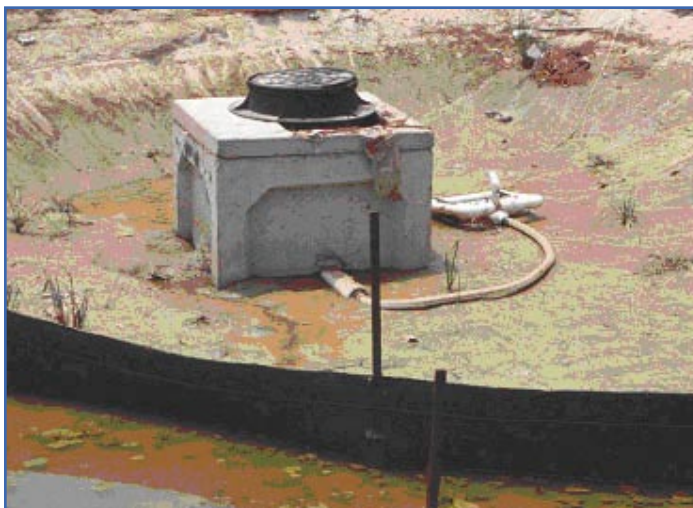
FIGURE 3. This sedimentation basin was converted to a bioretention cell at the end of construction. The concrete outlet was later utilized as the high-flow bypass. The slow draw-down skimmer was attached to the concrete structure in the same location as the bioretention cell's underdrains.
